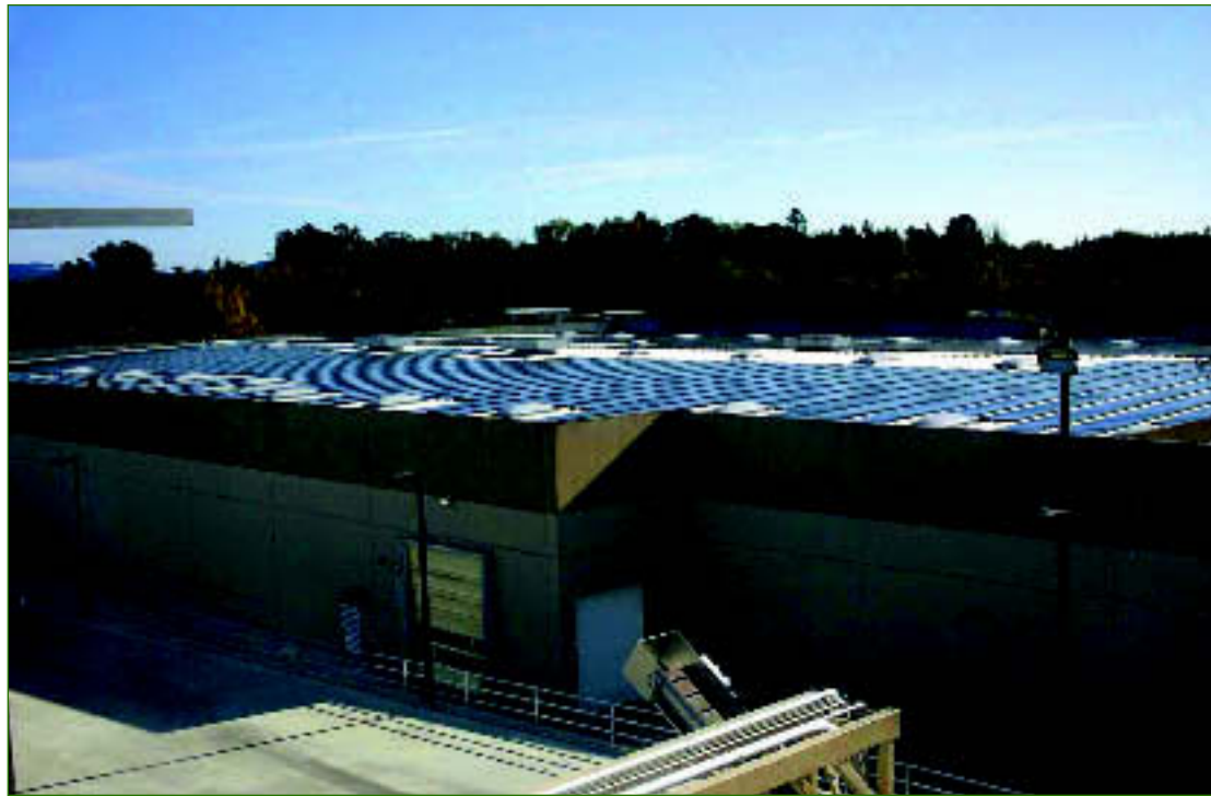
About 55 percent of the total roof surface is covered by PV modules producing 766,000 watts of DC power.
